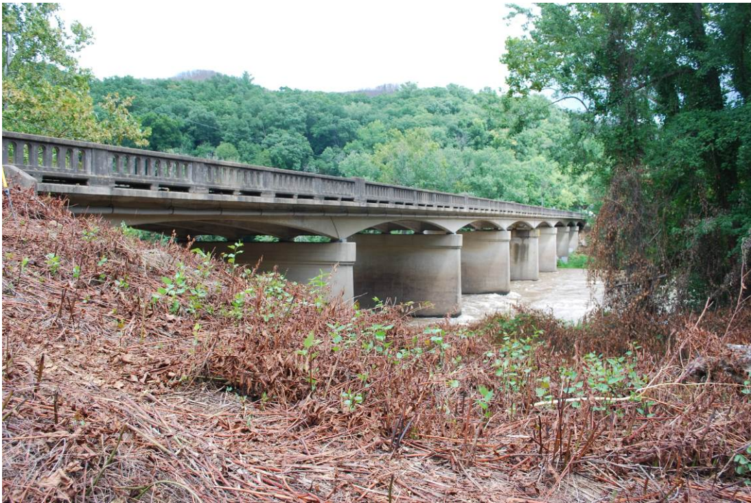
Photograph 4. Northeasterly View of Bridge No. 67 from the West Bank of the French Broad River
