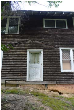
Photograph 32. Rear Elevation, Ghost Marks of former Gabled Porch
